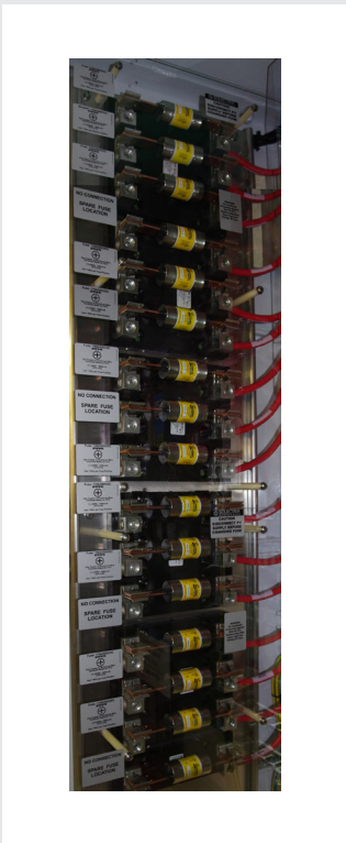
SGL 500 with 16 fused positions, 4 - 150A fuses, 4 - 125A fuses, and 8 - 175A fuses
