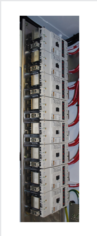
SGL 500 with 8 breaker positions, 7 - 400A breakers, and 1 - 350A breakers
